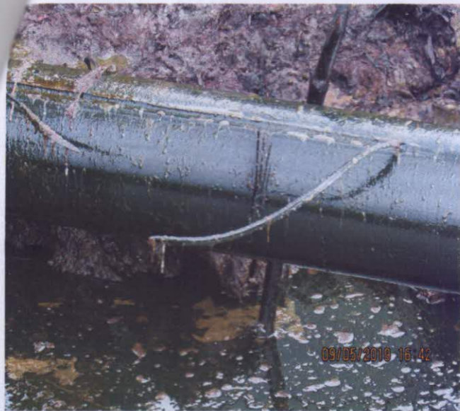
Figure 1: Hacksaw cut on the pipeline.
