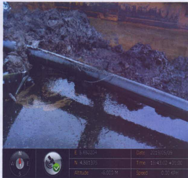
Figure 2: Hacksaw cut on the pipeline.
